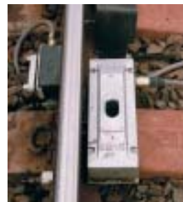
Above Reliable trains depend on reliable and up-to-date data. This is one of the electronic sensors that collects wheel temperature and other data as the train passes over. The data is transmitted immediately to the traffic-control centre in Port Hedland.
