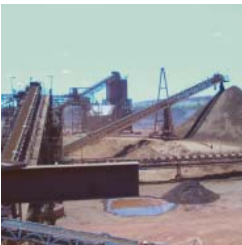
Above Orebody 25 view looking south from the apron feeder towards the main conveyor and bin loader.
